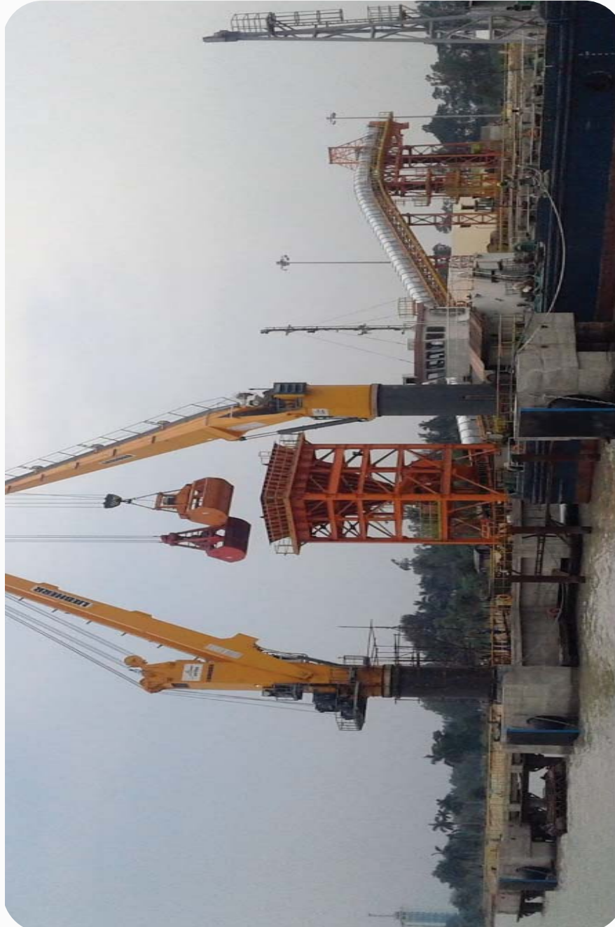
Floating Jetty - HDC
