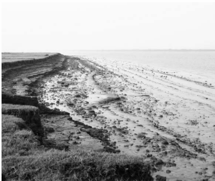
Erosion at Shalukkhali
